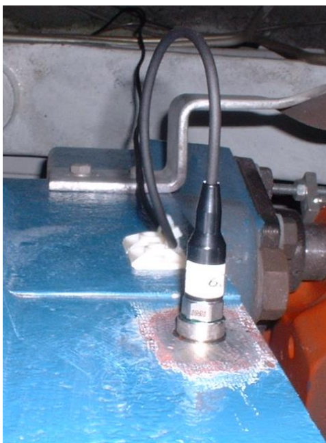
Picture 23: Vibration acceleration sensor glued on a mounting base
